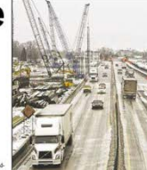
Construction workers are building the welcome center near the Port Huron area.
