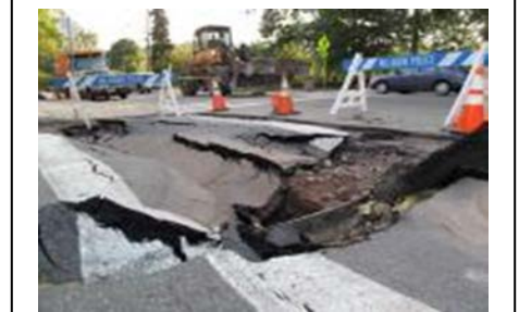
In this Sept. 2, 2011 photo, a front loader passes a sink hole in a Millburn, N.J. intersection. Officials say it could take months just to make basic repairs due to damage caused by Hurricane Irene. Many permanent fixes will have to wait until the spring. (AP Photo/Chris Hawley)
