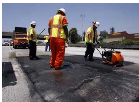
Caltrans workers make emergency repairs on a crumbling cement slab on Interstate 10 in Yucaipa in June. Caltrans says the inability to keep up with preventive maintenance on Inland roadways can create bigger, and more costly, problems later.
