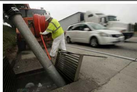
Caltrans' Paul Morones cleans out a drain along I-10 in Upland last month. Recent road failures have been attributed to culvert and drain difficulties.
