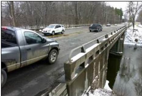
(ROD SANFORD/Lansing State Journal) Popular byway: Traffic moves Monday on Hagadorn Road over the Red Cedar River in East Lansing. Some 27,600 vehicles per day pass over this bridge, which is rated one of the most structurally deficient in the Lansing area. The bridge was built in 1930.
